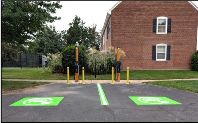
Brand new to the Glen - EV charging stations have been installed in Court 7 for Glen residents/guests.
